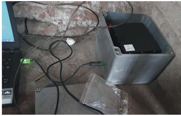
Figure 5. Sensor S.2 at level +37 m inside the tower.
