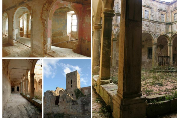
Fig. 2 – Details of inside of the Camaldolese Monastery before the last restoration activity (Copyright: ArTeSalVa project)
