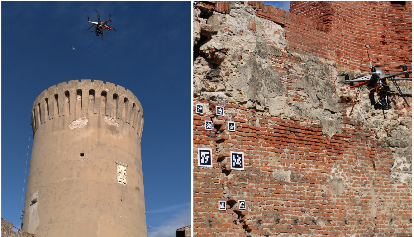
FIGURE 5: The two main different tasks of the UAV in the proposed IoT system: on the left, image acquisition for 3D reconstruction; on the right, periodical image acquisition for marker-based structural defects monitoring.
