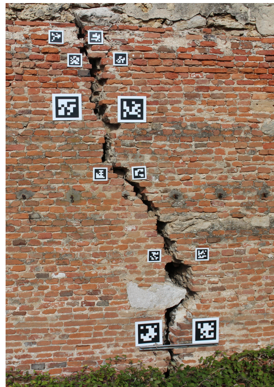
Figure 2: ArUco fiducial markers have been placed along the crack in the most critical points.
