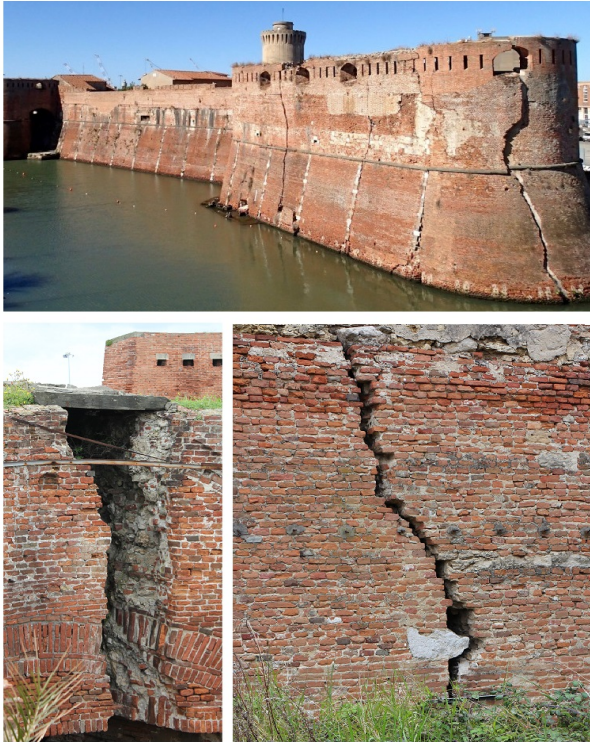
Figure 1: Evident structural defects in the walls of the ancient fortress, in the area named Bastione della Capitana (Fortezza Vecchia, Livorno, Tuscany, Italy).
