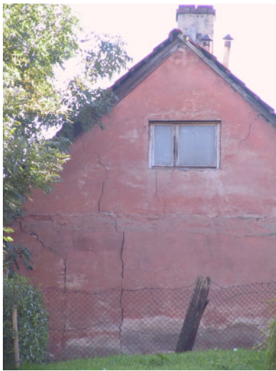
Figure 7. Examples of distressed buildings situated near the main square of Wieliczka.
