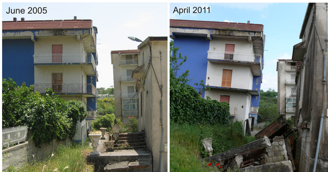
Fig. 7 Photo comparison showing an increase during the analysis period of tilt angles of buildings located on the edge of the landslide slope in the area of San Leonardo
