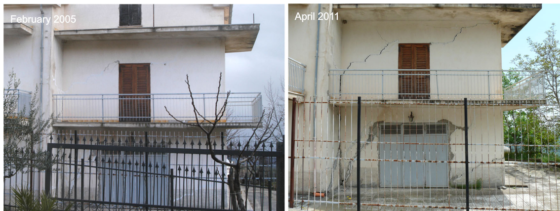
Fig. 6 Photo comparison showing an increase during the analysis period in the crack pattern of a building located in the Cemetery area
