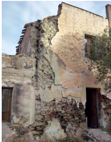
Fig. 6 Medau Palatini, Is Lois, Santadi (SU), detail of exterior of building before restoration (Photo Marco Bianchi)
