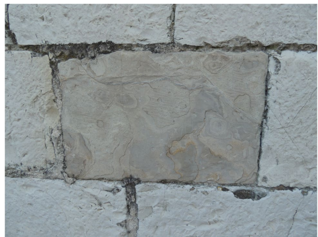
Fig. 8 Slight exfoliation developed when the ashlar is laid perpendicularly to the stratification
