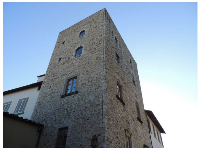
Fig. 15 Tower house of Villa San Lorenzo (fourteenth century) in Sesto Fiorentino (Florence)
