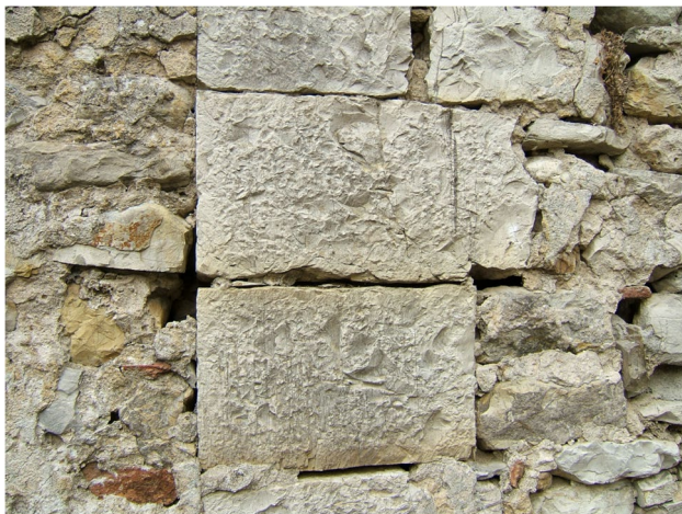
Fig. 1 Pietra Alberese ashlars with evident conchoidal fracture in a country house near Sesto Fiorentino (Florence)
