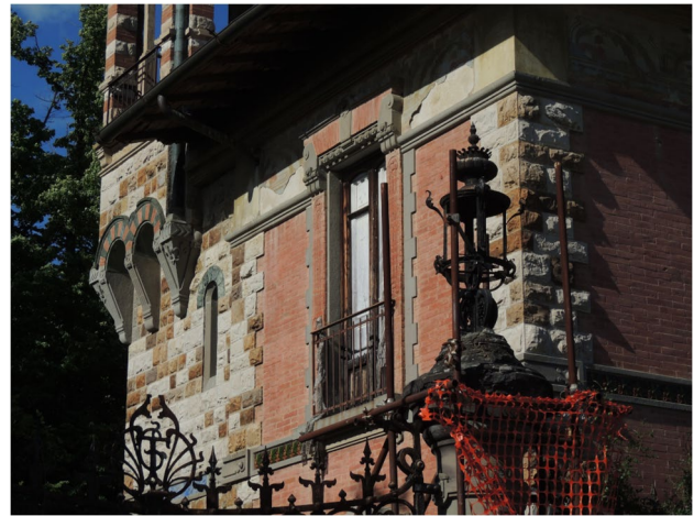
Fig. 26 Rusticated Alberese ashlar in the cornerstones and in the masonry of the access buildings to the Villa Peragallo in Calenzano Castello (Florence)
