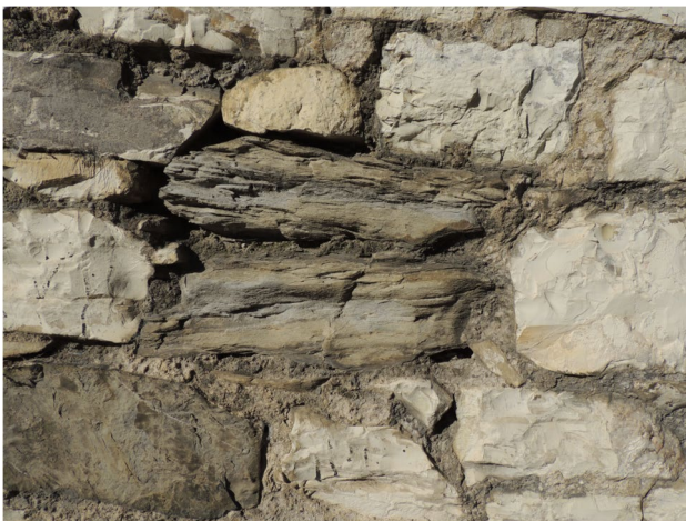
Fig. 10 Decay developed through 'soap' flaking in an ashlar realized from more marly beds of Pietra Alberese
