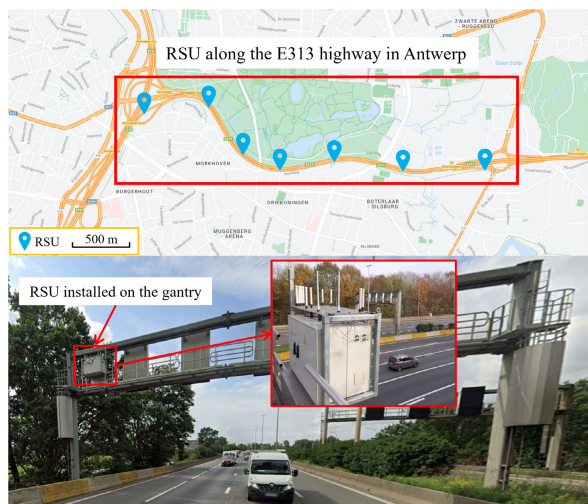
FIGURE 4. RSUs deployment along the E313 highway in Antwerp (upper) and RSU used for measurements and its installation position on the top of a gantry (lower).
