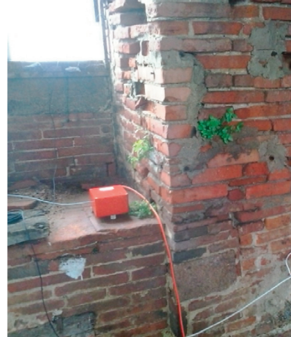
FIGURE 5. A SARA seismic station installed on the bell chamber.
