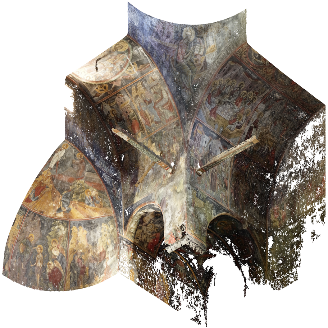
Fig. 10. The point cloud from the close-range photogrammetry process illustrates the vault's geometric complexity and decorative richness.
