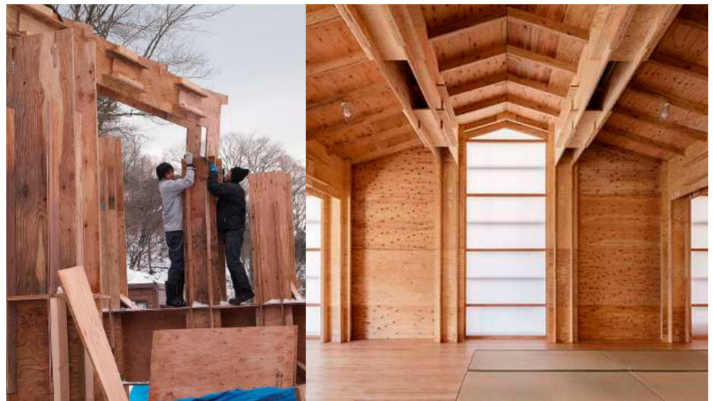
Figure 18. Veener House assembly process and final result. The wood components are designed to be lightweight and easy to assemble, in order to be joined by non-specialized workers and volunteers. Courtesy of Hiroto Kobayashi/kmdw.
