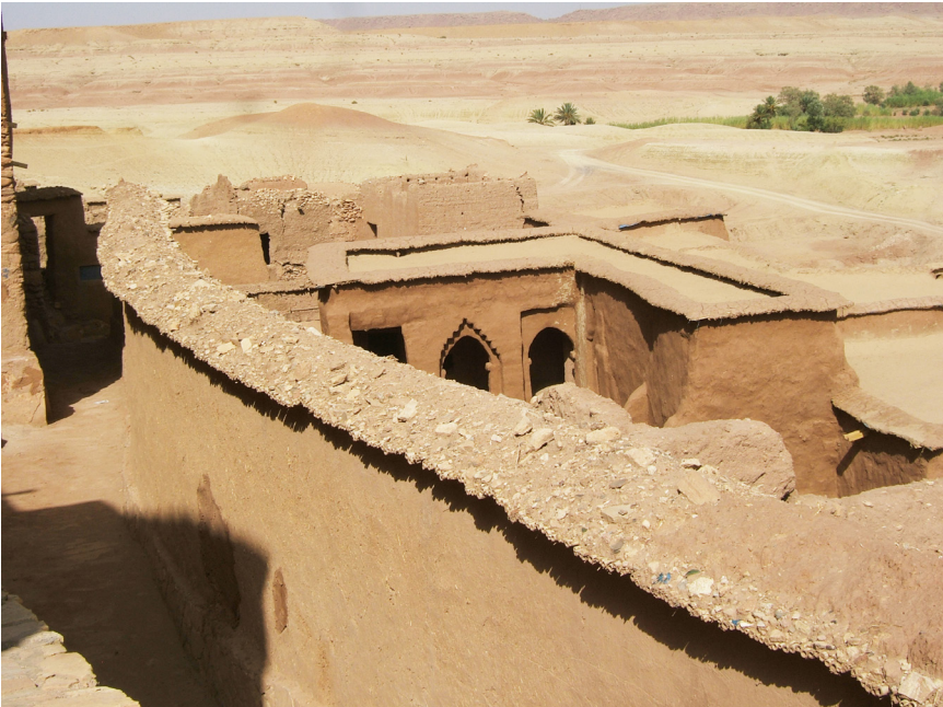
Fig. 9 Protection of the ridge of the walls to avoid water infiltration (Morocco)
