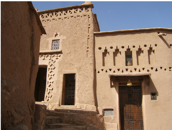
Fig. 5 Accurate maintenance of houses in the village of Ait Ben Haddou (Morocco)
