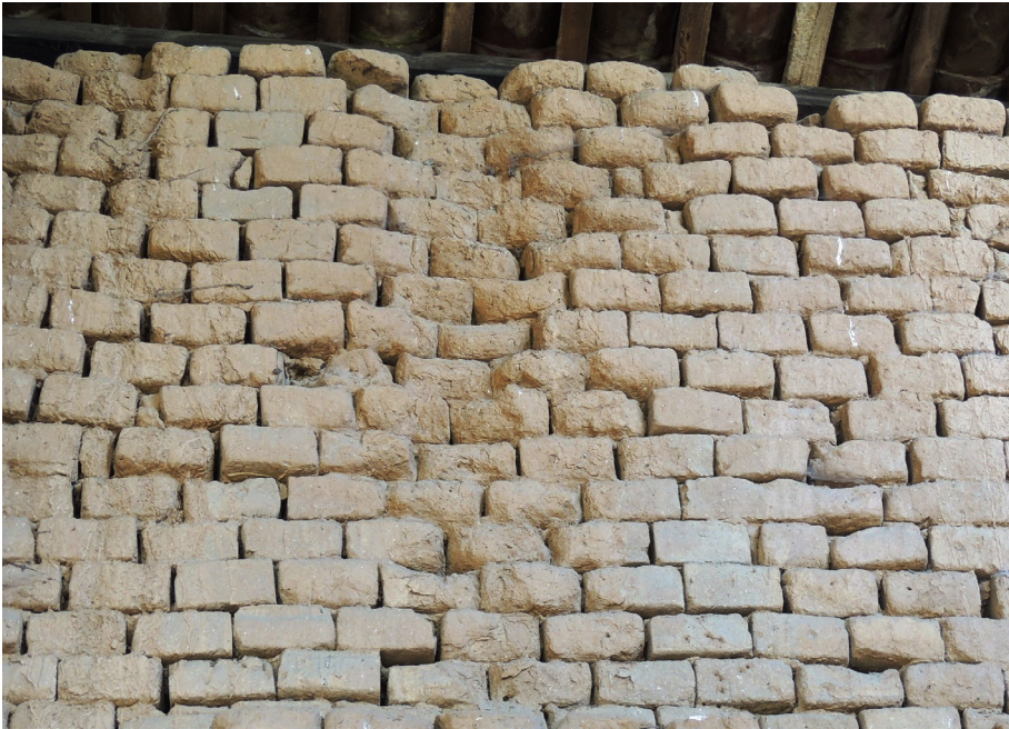
Fig. 4 Rain erosion of an adobe masonry in Piedmont (Italy) due to lack of maintenance of the roof
