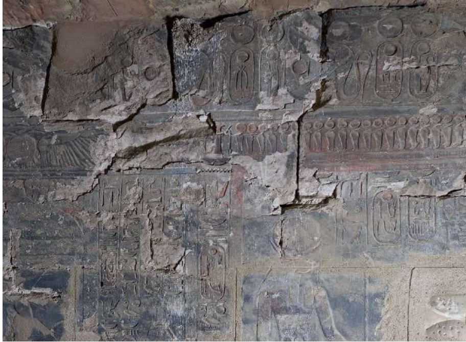
Fig.15 - Room X, structural problems - photo by C. Vazio
