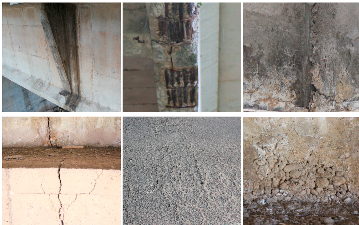
Fig. 1. Defect typologies investigated. From the top to down and from left to right, the following defects can be recognized: moisture spot, corroded steel reinforcement, deteriorated concrete; cracks; pavement degradation; honeycombs.
