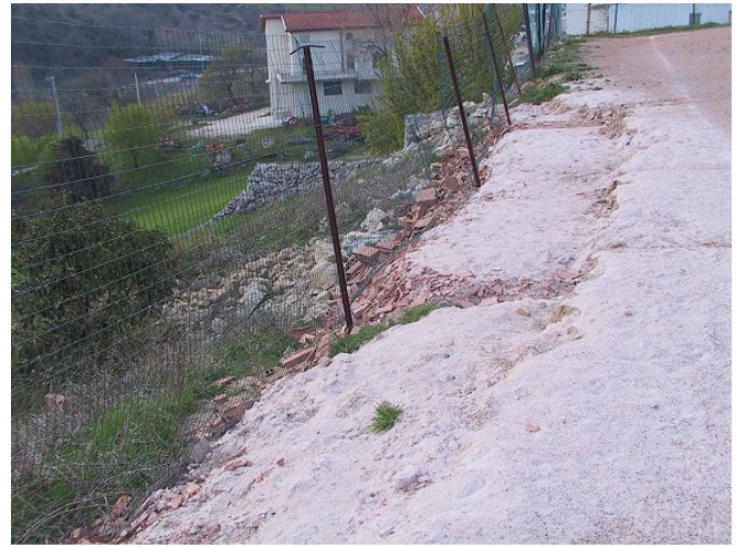
Figure 6. Small rotational slide at the SW corner of Pietramontecorvino football field, whose movements were detected by PS interferometry (cf. Fig. 5). Note semi-circular scarp with minor ground settlement.
