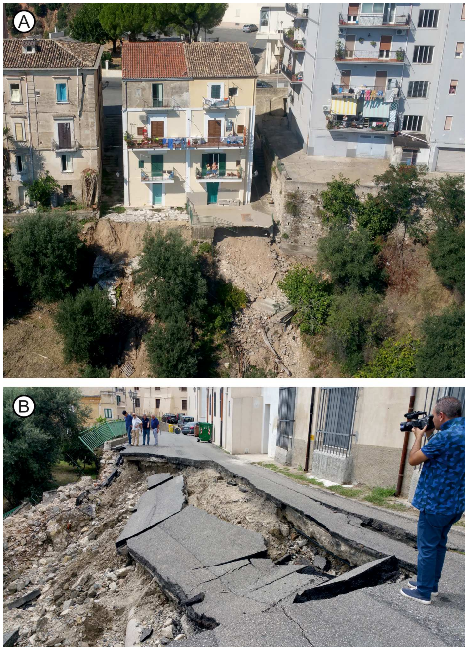
Figure 7. Landslides that occurred in Corigliano-Rossano town during the flood event of 12 August 2015. Historic centre of Rossano: (A) Vittorio Emanuele road, (B) Via Minnicelli road.
