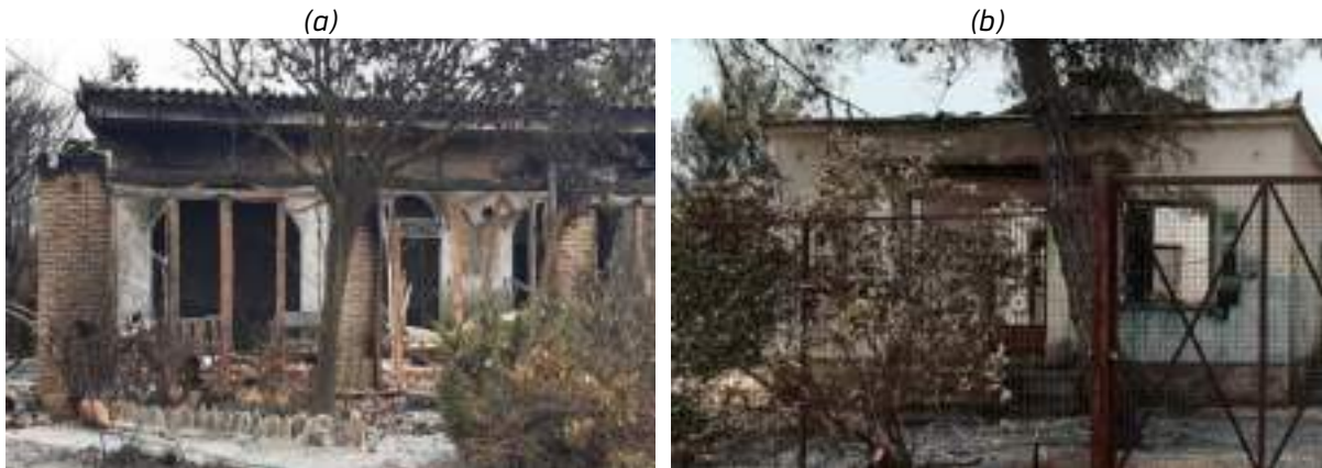
Figure 82 – Damage due to fire entrance by openings in isolated houses in Tatoi settlement (NKUA Newsletter)[24].
