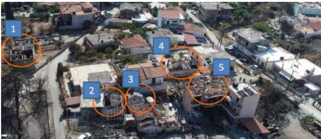
Figure 104 – Fire-induced roof damages identified by UAV flight performed by the University of Athens (Source: NKUA Newsletter., 2021) [24].
