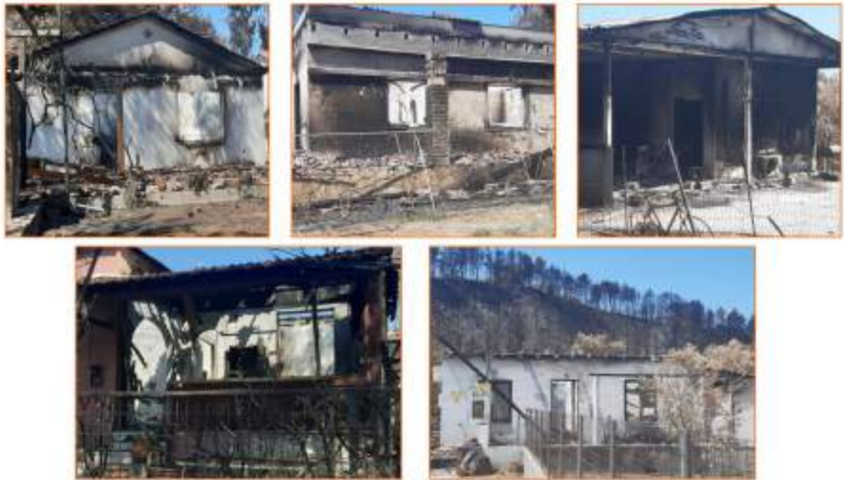
Figure 105 – Fire-induced damage due to aged and old building material (Source: NKUA Newsletter., 2021) [24].
