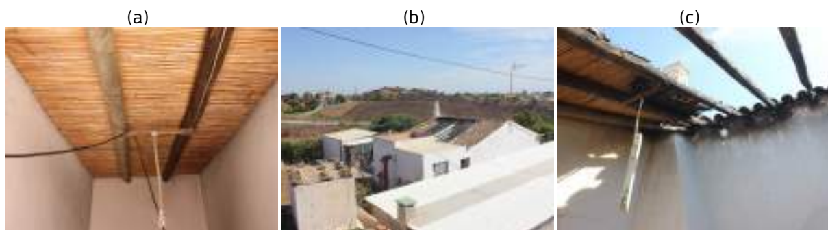
Figure 29 – Images regarding the case study of Corte António Martins: a) photograph of a reed roof; b) general image of the house where is possible to see the roof area that was damaged by the fire; c) indoor image of the roof that was damaged by the fire, where we can see the reed roof where the fire started.
