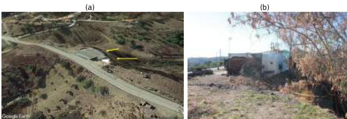
Figure 21 – a) General view of the building damaged – the yellow arrows indicate the provenience of the fire front; b) photo of the back of the building where it is possible to see the proximity of forest fuels such as trees.
