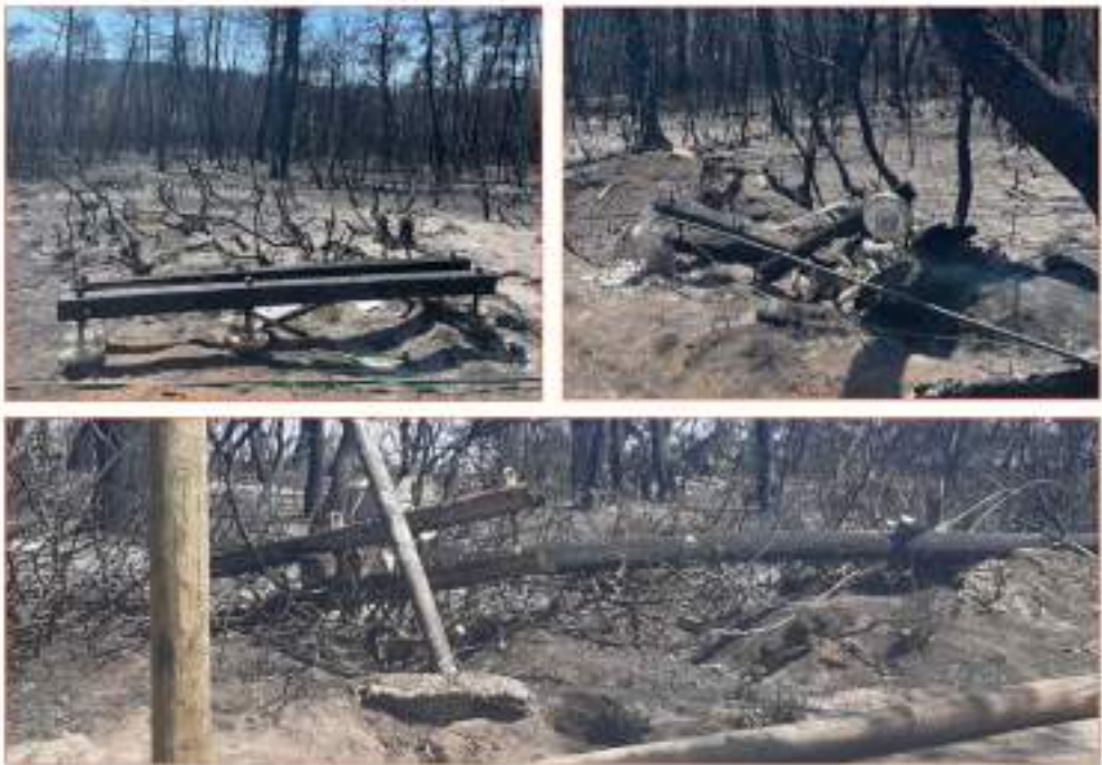
Figure 106 – Damage to the power distribution network in Ayia Anna (Source: NKUA Newsletter., 2021) [24].
