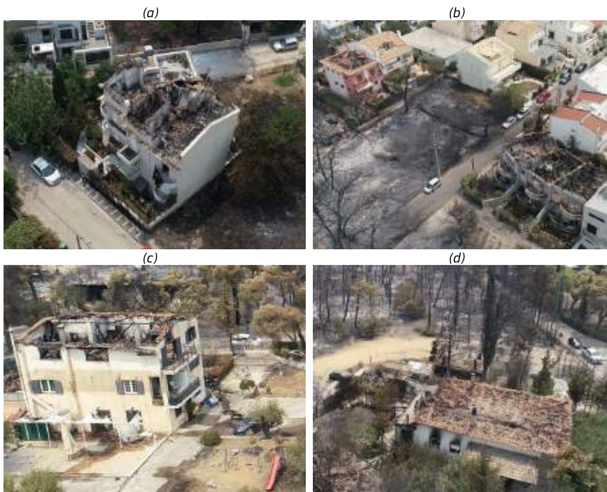
Figure 81 – Collapsed roofs and burned house interior in building blocks in a) and b) Adames settlement (NKUA Newsletter); c) and d) Tatoi settlement (NKUA Newsletter)[24].
