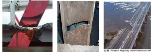
(a) Damage point for repair (b) damage point for repair (c) Damage point
