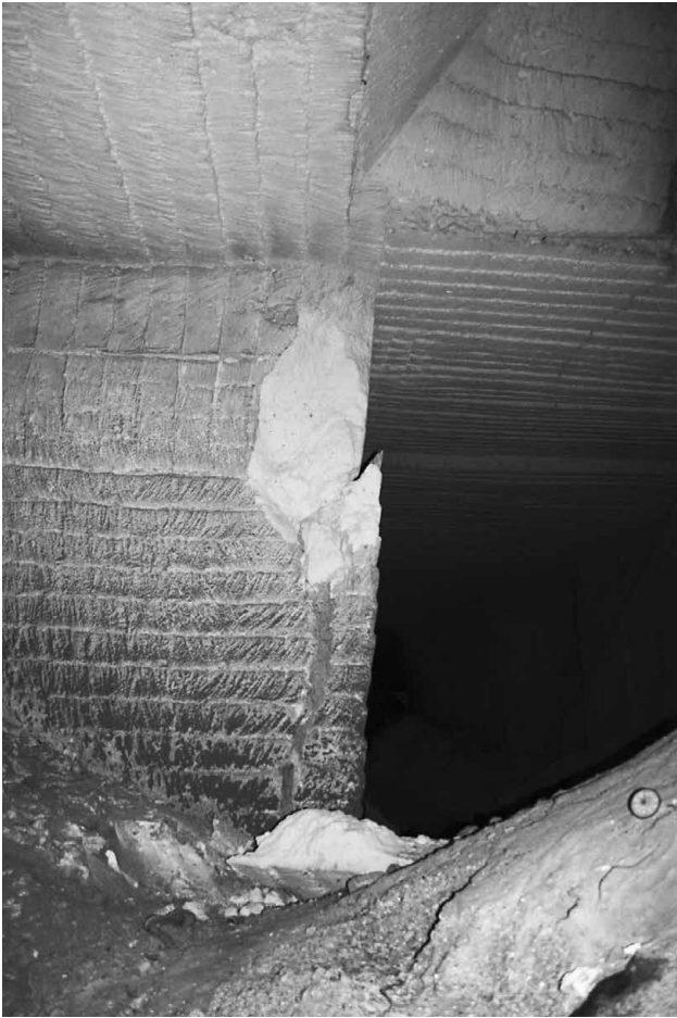
Figure 3. Failure at the upper corner of the pillar.
