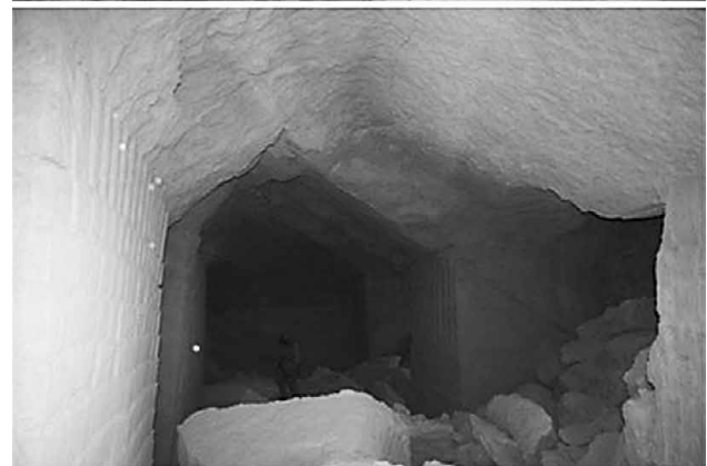
Figure 9. Double (above) and single (below) arches produced by failures at the vault.
