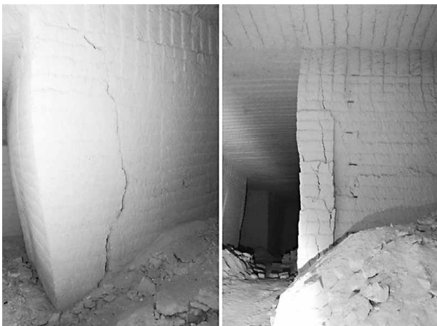
Figure 6. Examples of cracks developing at the pillar corners.
