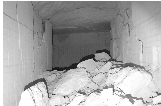
Figure 1. Massive fall from the vault in a calcarenite quarry.
