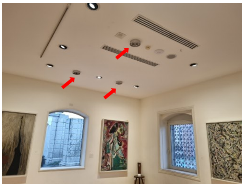
Figure 2. Room PG-5. Red arrows indicate the exact position of sampler racks with passive samplers.
