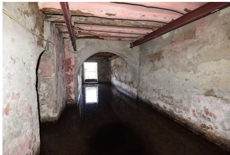
Figure A11. Flooded ground floor in a building along the coast of Marina Lunga. Until the 1980s, it was used as warehouse, but later, it was abandoned due to sea level rise. Presently, the ground floor is below the local sea level.
