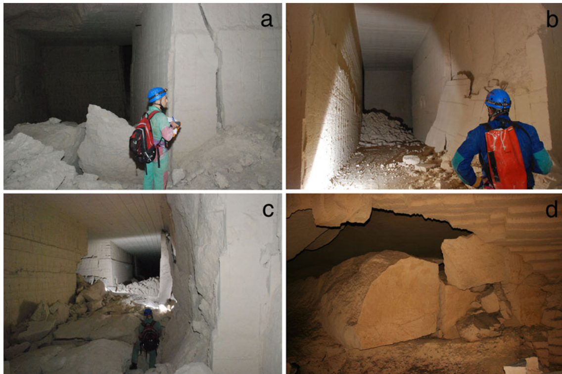
Fig. 4 Failures in underground quarries, potentially leading to upward stoping of instability and development of a sinkhole at the ground surface. a Open cracks in the pillars and falls from the vault
