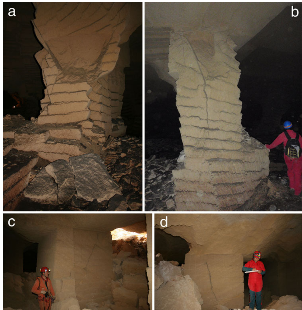
Fig. 6 Examples of pillars with open cracks and deformations in underground quarries of Apulia: a, b detachment ( a ) and open cracks ( b ) in pillars at Gallipoli; c, d open and crossed cracks in pillars at Barletta
