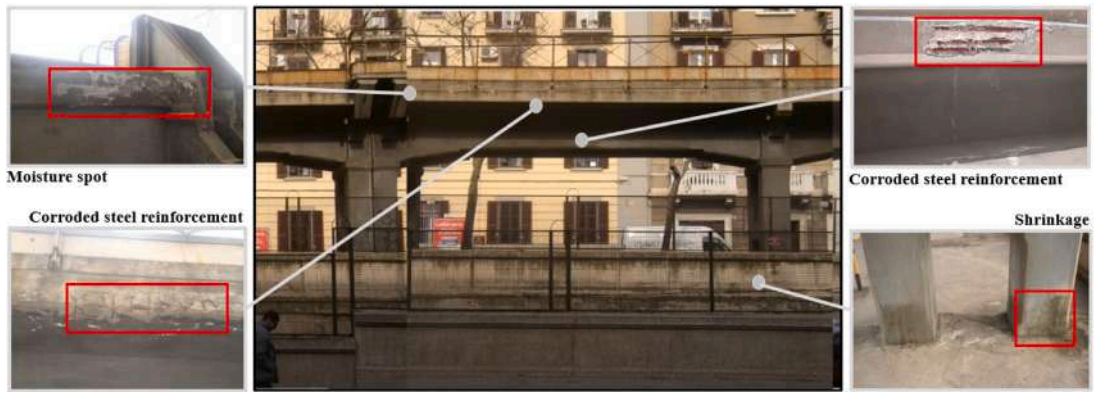
Fig. 16. Typical defects manually detected on a bay of Viaduct of Corso Italia. Red boxes indicate the damage box for each image.
