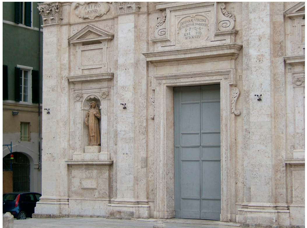
Figure 7. The travertine cladding of the façade of Santa Maria di Provenzano (Siena, XVIIth century) (credit Fabio Fratini).
