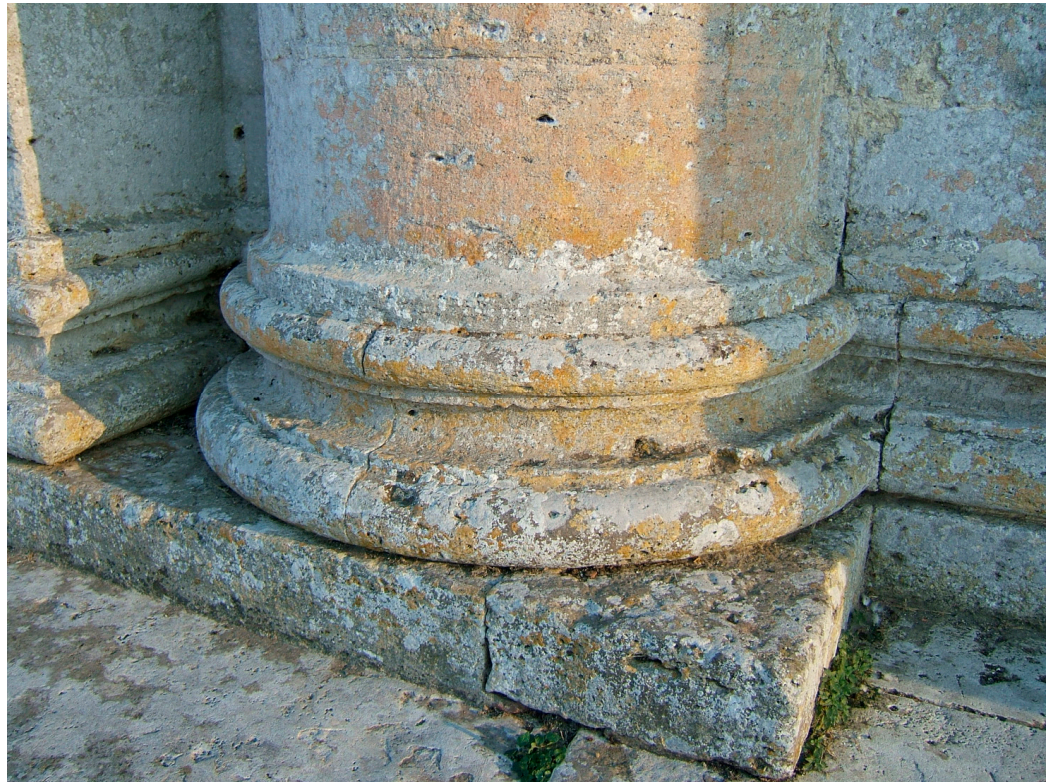
Figure 24. Growth of lichens on the travertine architectural decorations of the Church of San Biagio in Montepulciano (credit Oana Adriana Cuzman).
