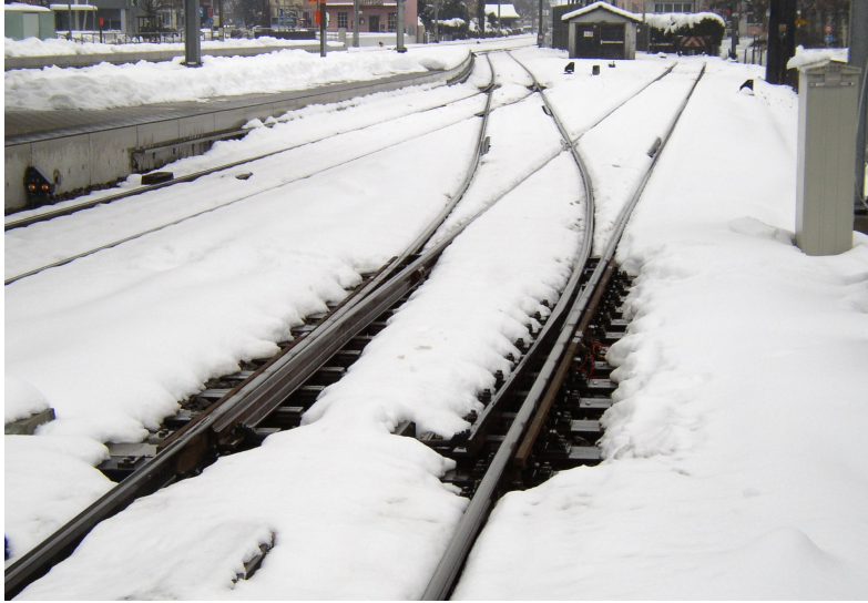
Fig. 1. Gas heating keeping a railroad switch free from snow and ice (Di Fabian Grunder (FabiBerg) – Opera propria, CC BY-SA 3.0, https://commons.wikimedia.org/w/index.php?curid=641923 )
