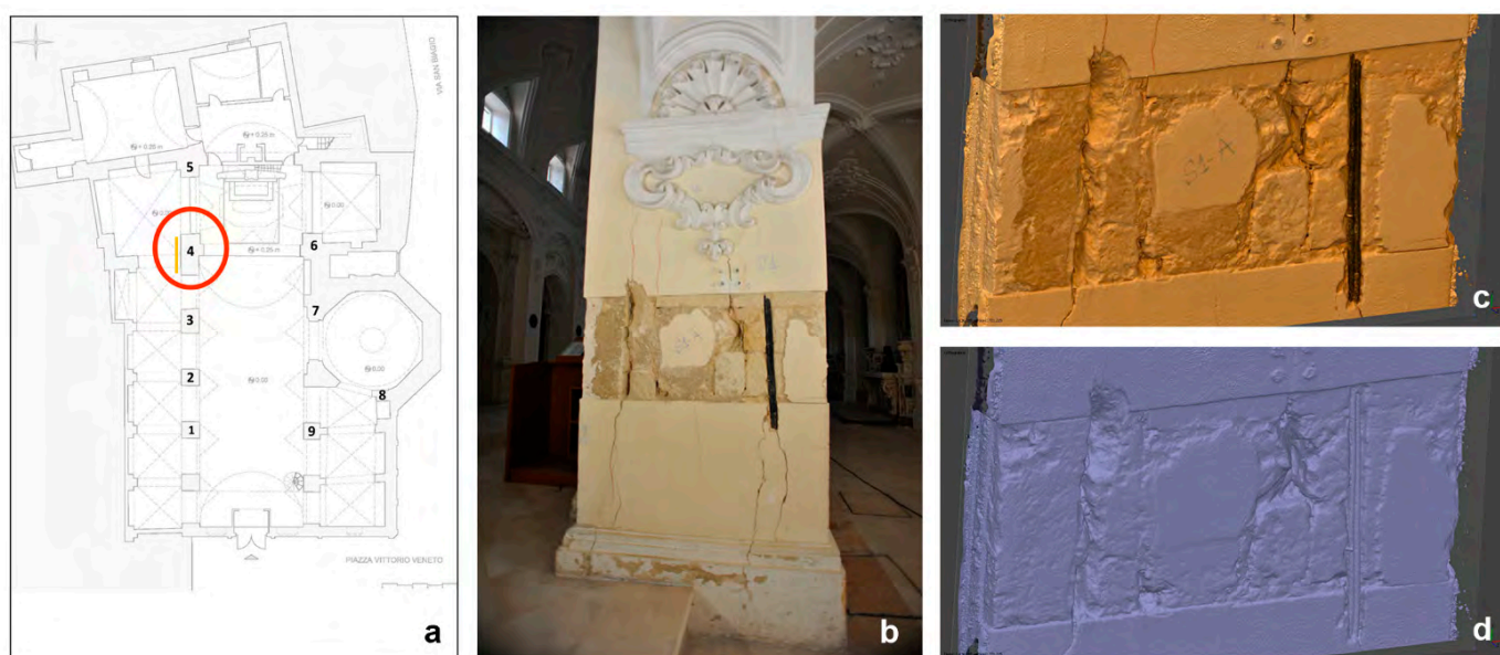
Figure 6. Photogrammetric processing of the lesion present on pillar nr. 4. General plan of the Church (a). Image of the lesion (b). Various views of the lesion (c,d).
