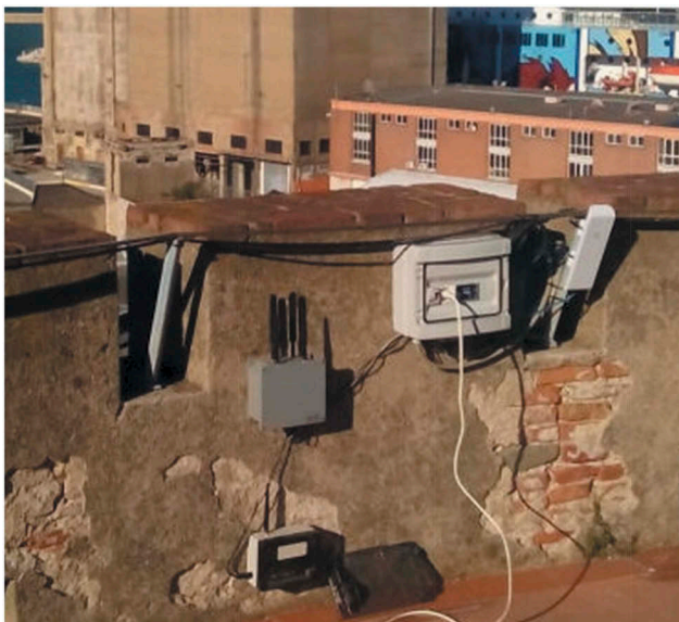
Figure 2. View of the gateway (installed on the tower case study).
