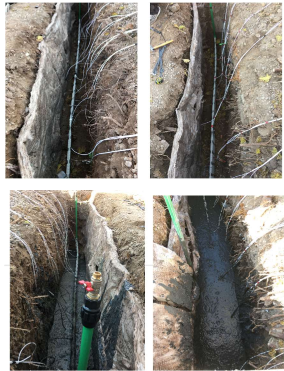
Figure 5: Flat heat exchangers with sensors and grout material
