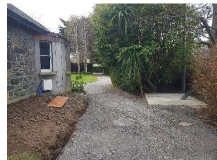
Figure 8: Drilling at the Greystones demonstration site and location of the new plant room to accommodate the dual cycle heat pump.
