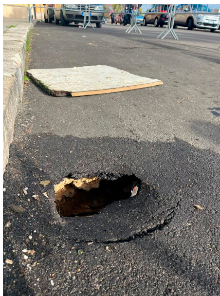
Figure 4. Collapse phenomena in late December 2022.
