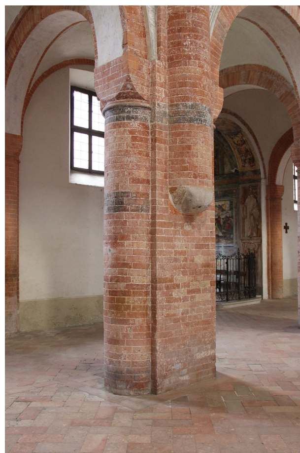
Fig. 17 | Column in Cerreto a Lodi. The walling is done with very narrow joints of just a few millimetres. The individual bricks are also made with precise, right-angled edges. The pillars in the nave of the abbey church have no plinths that could be hidden under a raised floor (Photo: Thomas Bertelsen).
