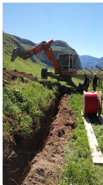
Figure 10. A trench dug at the downstream toe of a levee for the installation of the optical fibre cable (visible at the right) for a Raman-DTS monitoring campaign.
