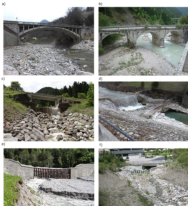
Figure 3. Photo record of the structures inspected: (a) upstream view of bridge 1: pretest and test 1. (b) Upstream view of bridge 2: test 2. (c) Upstream view of bridge 3: test 3. (d) check dam 1: pretest and test 1. (e) Opening of check dam 2: test 2. (f) Upstream to downstream view of check dam 3: test 3.
