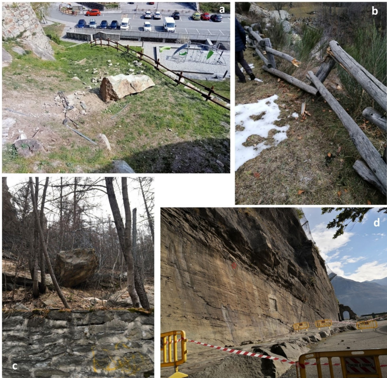
Fig. 9 (a) Rockfall occurred in correspondence of the footpath to the Fort of Bard, renowned tourist site; most blocks have obstructed part of the path, while a block of 3 \text{ m}^3 has broken through the parapet on the valley side, reaching the area close to a parking (EDF cod. 36421); (b) Wooden fence of a footpath destroyed by a rockfall event that involved the gabions on the valley side, Perloz (cod. 36660); (c) Rockfall occurred upstream of the track of a cement factory, with a block of 1.5 \text{ m}^3 intercepted by the existing rockfall barriers, Courmayeur (cod. 35927); (d) small blocks fallen along the “ Strada Romana delle Gallie ”, a renowned footpath to the archaeological site of the Roman Arch, Donnas (cod.35863), the event occurred just below the nets and the rockfall barriers
