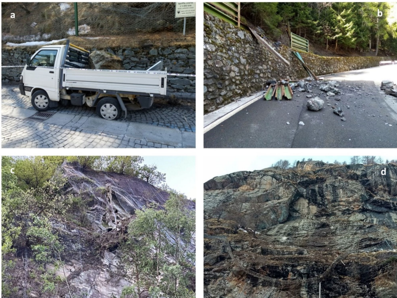
Fig. 7 (a) Damage to a rockfall barriers along a municipal road, a block of about 0.7 \text{ m}^3 hit a vehicle causing serious damage, Cogne (EDF cod. 34933); (b) metal rockfall barriers with horizontal elements place in the 90s to protect the regional road S.R.39 destroyed by a rockfall of about 1 \text{ m}^3 , Morgex (cod. 36135); (c) rockfall event of about 6\text{--}8 \text{ m}^3 causing the rupture of the mesh drapery system and interrupting the municipal road with severe damage to the road pavement, Pontey (cod. 36150); (d) rockfall barrier upstream a cheese factory completely removed for 30 m in length by a rockfall of about 30 \text{ m}^3 , Valgrisenche (cod. 36393)
