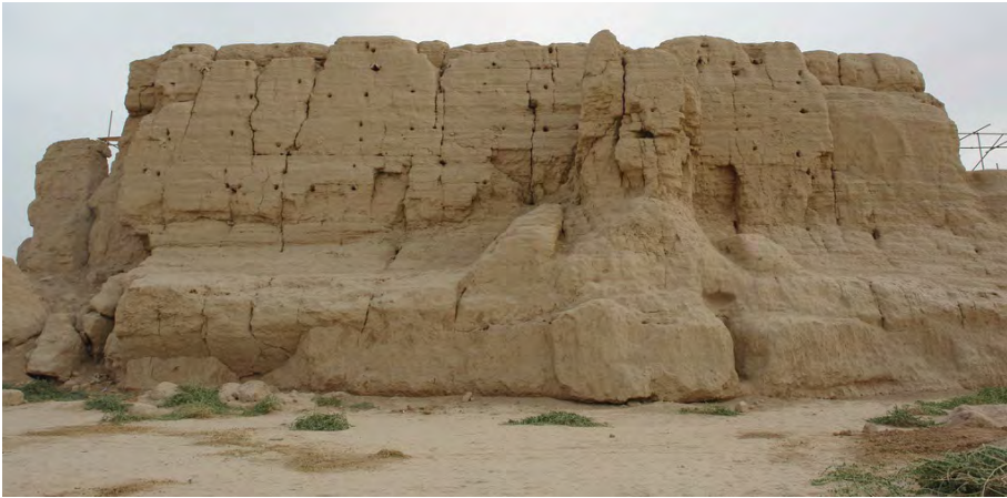
Fig. 7 General view of rammed earth walls before the construction of an adobe masonry support
