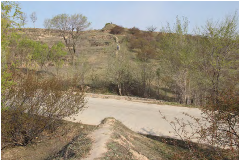
Fig. 9 An example of modern destruction, the Great Wall cut into two sections by a road
