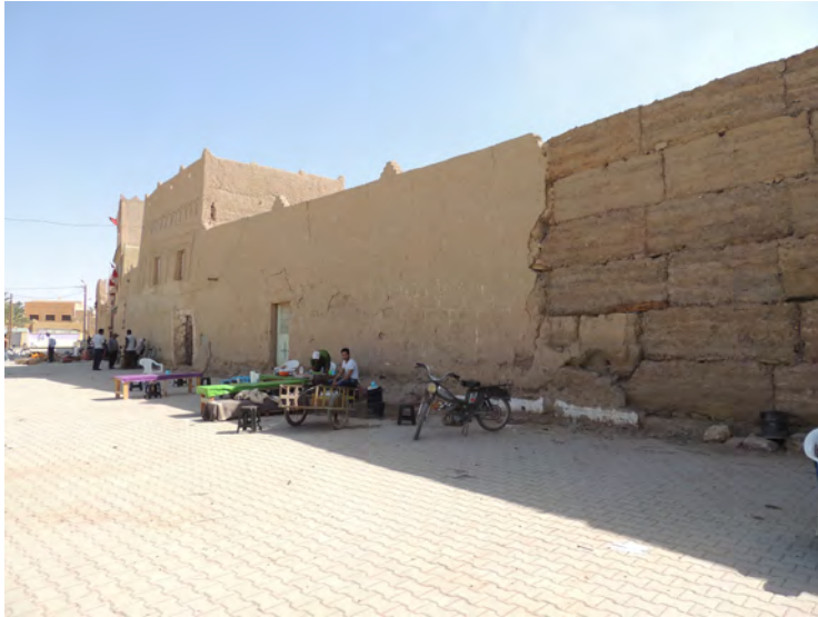
Fig. 10 Ongoing works to protect with an earthen plaster the walls of a village in Morocco
