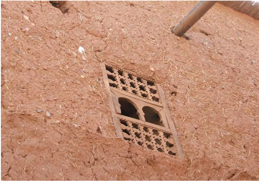
Fig. 6 Earthen plaster added with vegetable fibers to avoid shrinkage fractures (Morocco)
