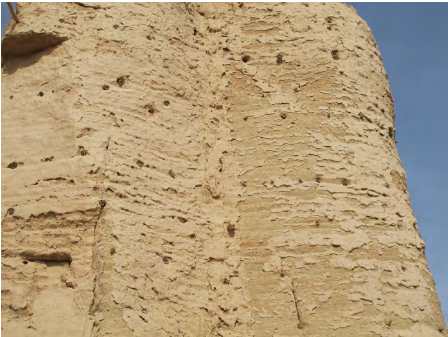
Fig. 2 Spalling decay effect on a wall
