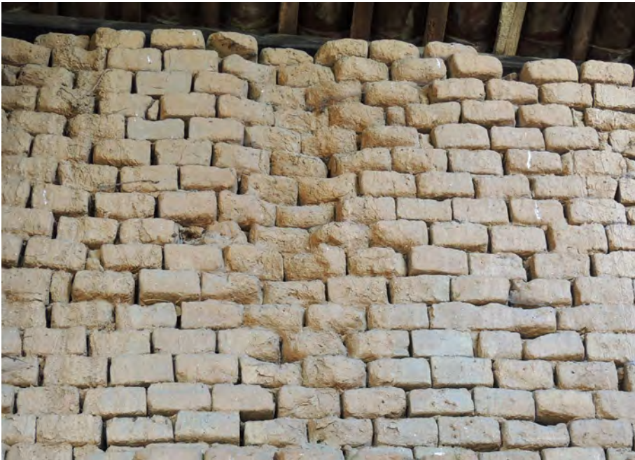
Fig. 4 Rain erosion of an adobe masonry in Piedmont (Italy) due to lack of maintenance of the roof
