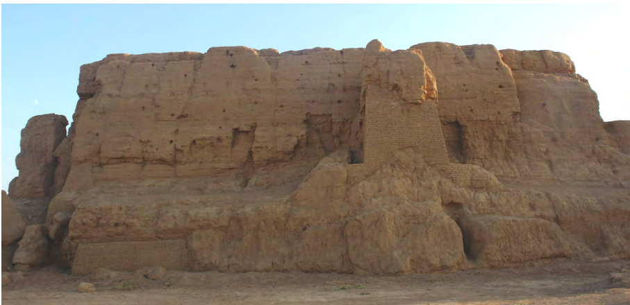
Fig. 8 General view of rammed earth walls after the construction of an adobe masonry support
