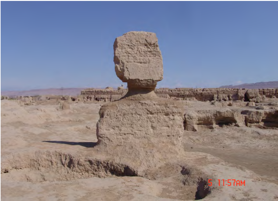
Fig. 3 Rammed earth wall eroded by winds
