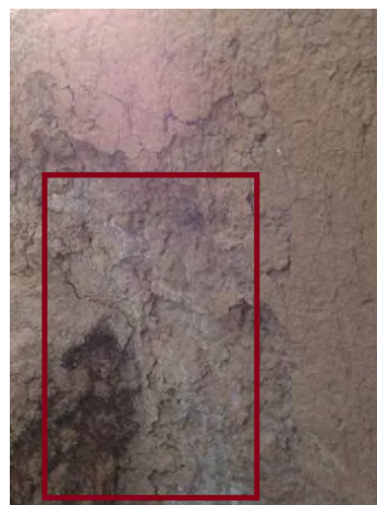
Fig. 4 Biodegradation caused by mould in area F29 (red square)
