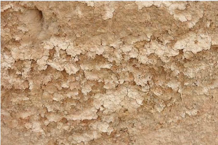
Fig. 5 Thin layer formed on the surface of an earthen wall after rain, subsequently cracked and about to fall
