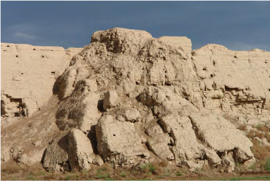
Fig. 2 Collapse of the rammed earth walls
