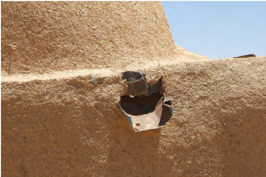
Fig. 8 Improvement of the water run-off to avoid concentrated flow on the walls in a Syrian corbelled dome house
