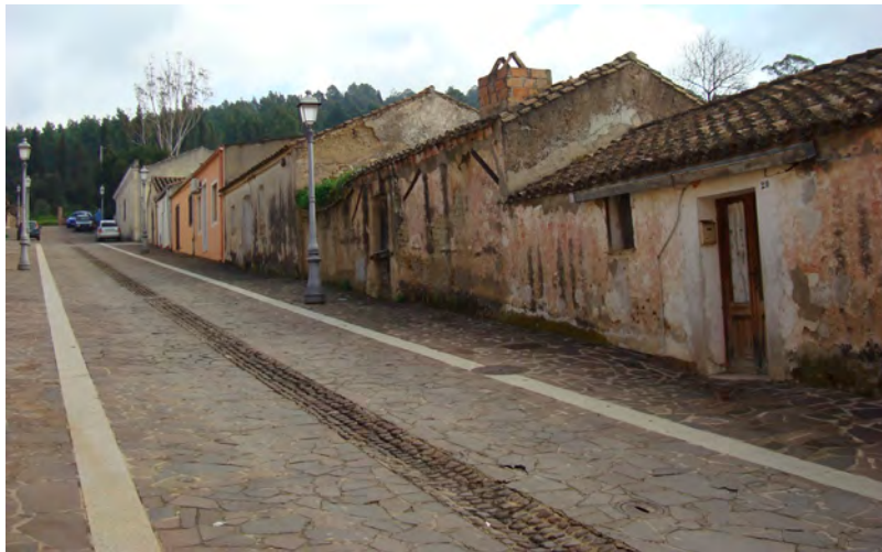
Fig. 3 Sa Domu 'e Pasci, Santadi (SU), exterior of building before restoration (Photo Paolo Paschi)
