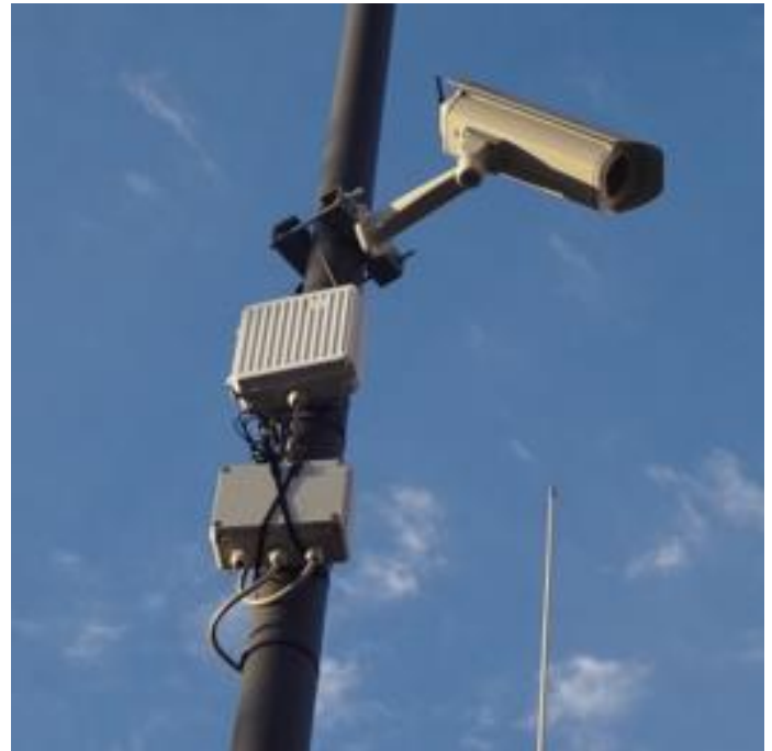
Fig. 7. An installed smart camera and the ETSI MSM Gateway installed on an existing pole during Montecatini trial
