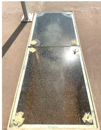
Figure 3. Dewing at the walkway showcase.
