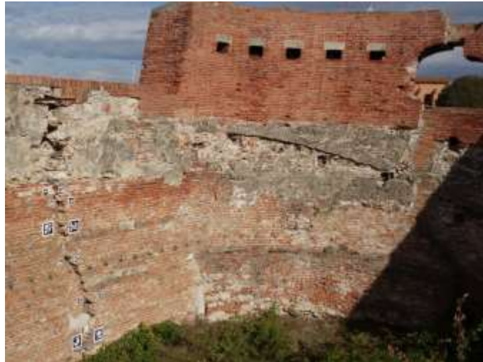
Fig. 3 – Bastione della Capitana. This area of the Fortezza Vecchia complex has been considered for long-term monitoring of cracks and damages in the building by UAV inspection. A configuration of markers has been placed around a crack to perform quantitative 3D measurements.
