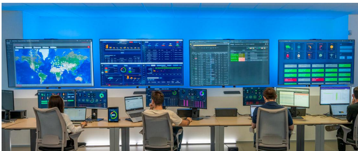
Fig. 11 A preview of the future Control Room configuration.
