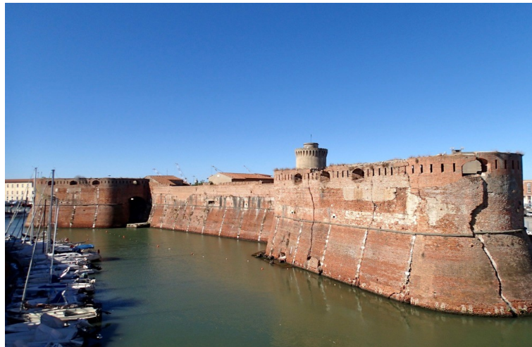
Figure 1. Fortezza Vecchia, Livorno, Tuscany (Italy). Evident structural defects can be noted on the walls of the ancient fortress (credits to Giacomo Spagnoli).
