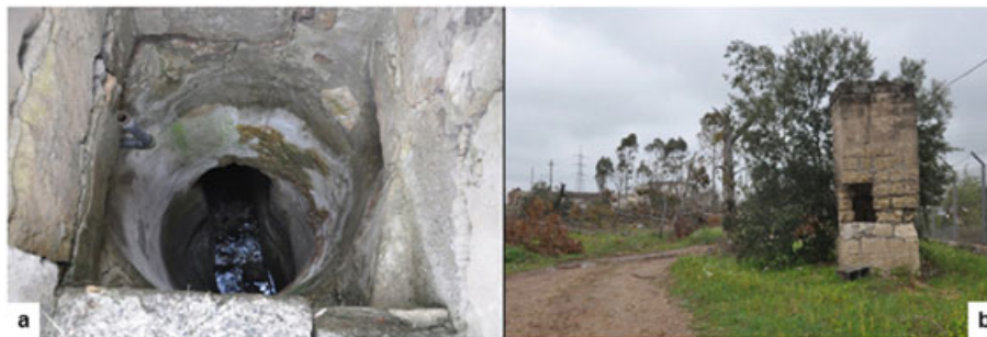
Figure 7. Shaft 1 with the underground tunnel (a) and the external structure of shaft 2 (b).
