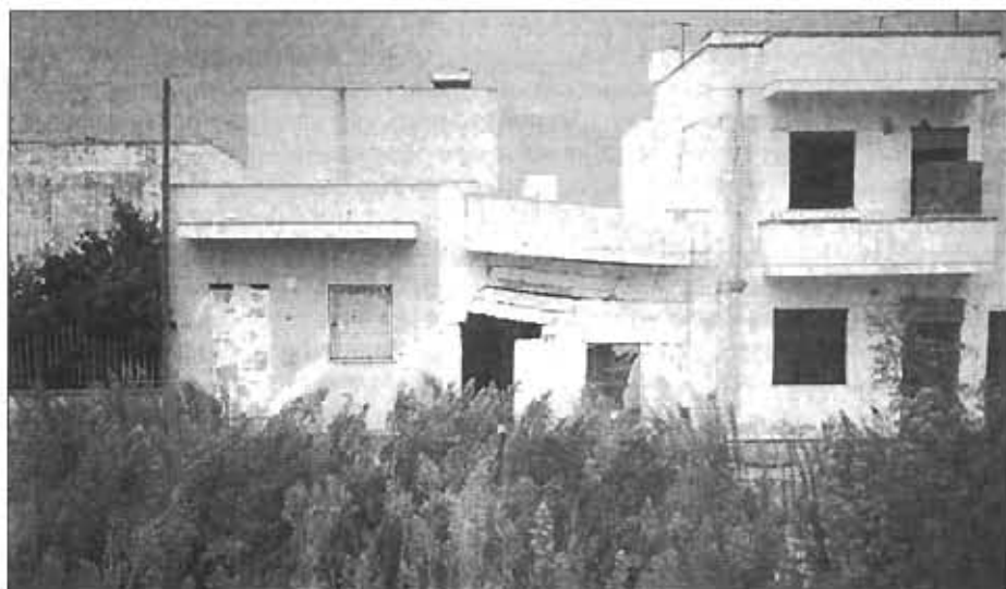
Fig.4 - Damage to buildings in the village of Casalabate, due to subsidence events that occurred in 1993 (photo taken in 1994).
