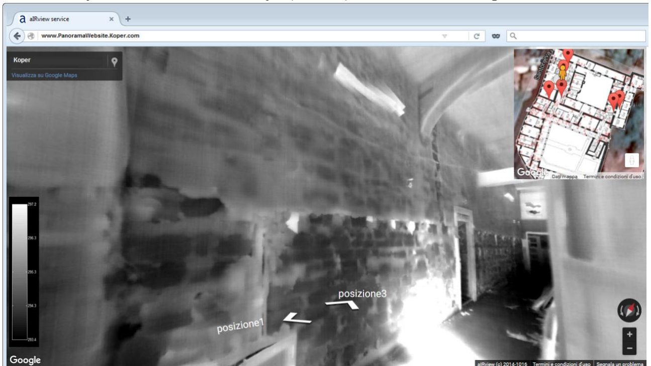
Figure 3. Thermal scan of the Servitski monastery in Koper. The different wall layout is highlighted by the thermal stimulus. The results are shown on a virtual visit of the building, where adjacent rooms could be easily compared [9].
