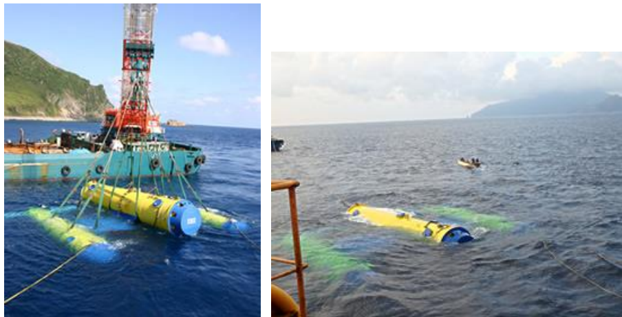
Figure 1: The preparation work for the demonstration test of the ocean current turbine “Kairyu” near Kuchinoshima Island (IHI and NEDO, 2017).
